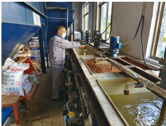
Waste Water Treatment in Action
