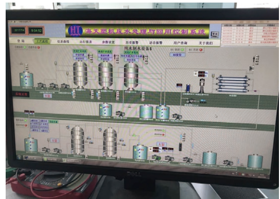
Waste Water Treatment and Reuse Control System
