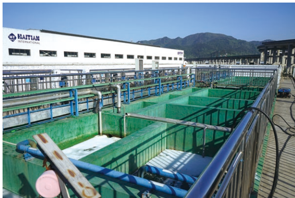
Rooftop Treatment Tank of the Waste Water Treatment Station
